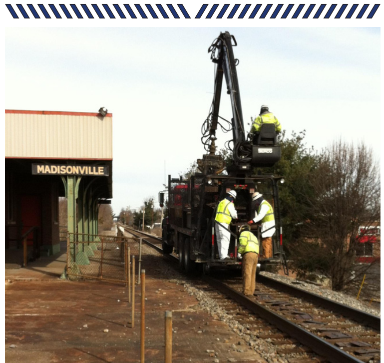
CSX drops rail plates in anticipation of replacing rail through Madisonville, KY with new and heavier rail. Dec. 28, 2014
